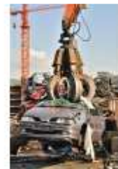
Scrap yard Method Statement and Risk Assessment
